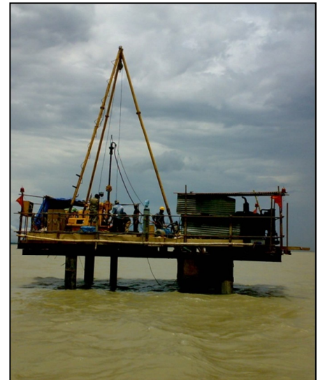
Drilling from Fixed Platform
